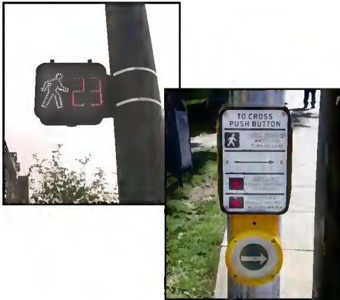
Audible Pedestrian Signal Push Button with Operational Signage
